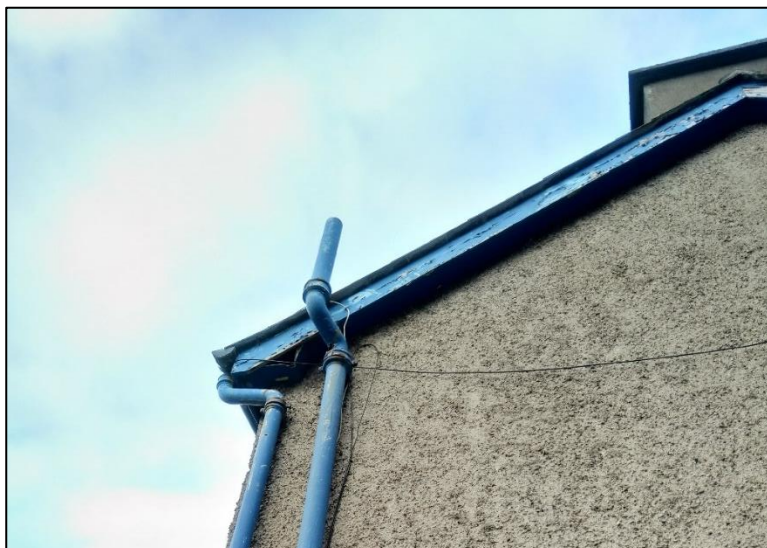
Figure 5. Photograph showing a hole in building eaves which may provide bat roosting habitat. Image taken 26/11/2020.
